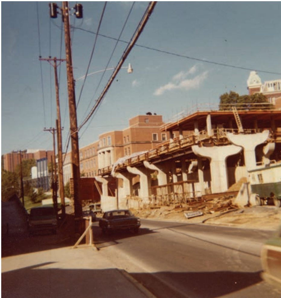
▲ Construction of Beechurst PRT station as seen from across Beechurst Ave. Summit Hall and Armstrong Hall in background. Top of Woodburn Hall visible on the far right. Circa 1972.
